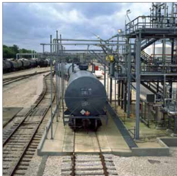
Figure 6.13 EO Unloading Facilities
