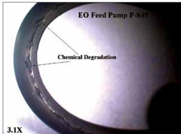
Figure 6.10 Example of Degraded O-ring Attacked by EO
