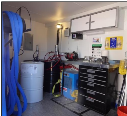
Inside Spray Rig
